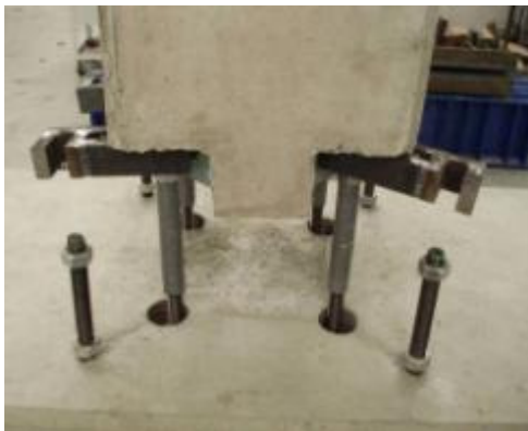
Figure 6 Inserting the threaded rods of the pillar in the plinth's ribbed hoses
